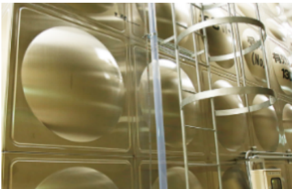
Daimaru Shinsaibashi water storage tank
